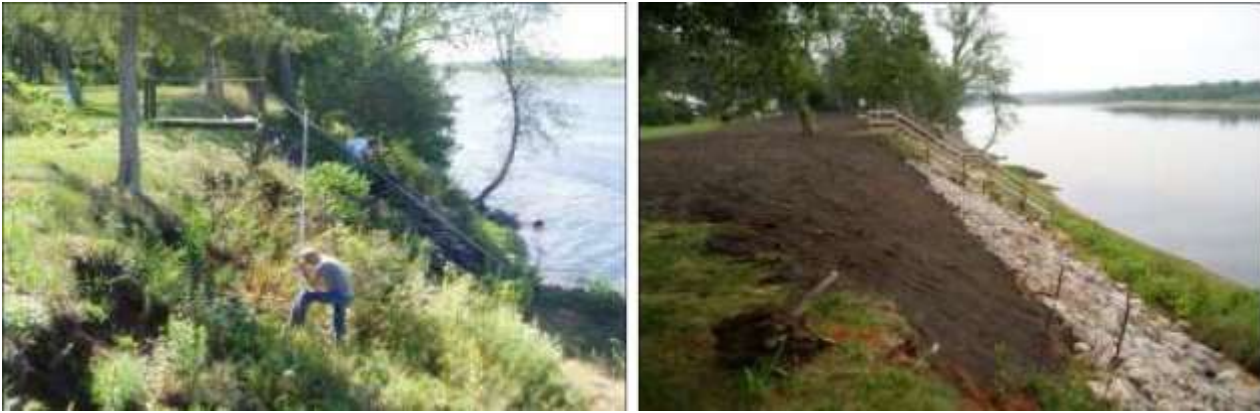
Before and after — installation of a streambank protection project along the Wisconsin River.
